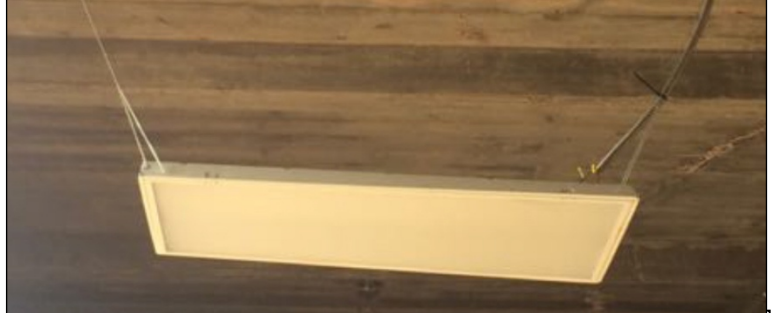
The fixtures were hung with weak chains, spread at precarious angles adding to the strain. Note the bare wires leading to the fixture. This needed to be fixed.
